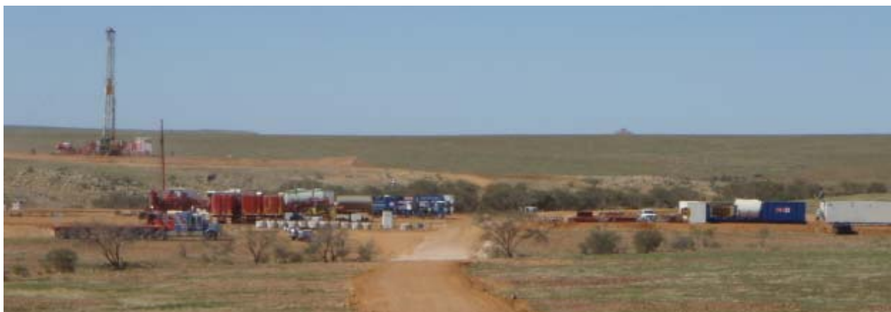
Workover rig and production activity on Flax field
